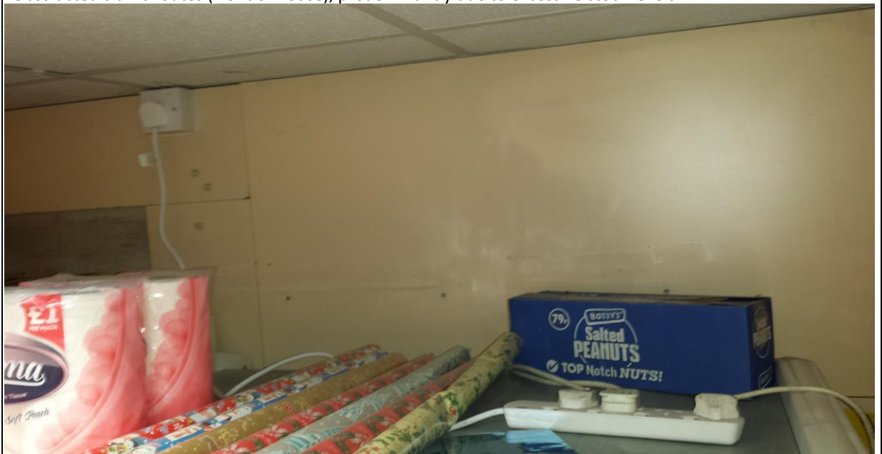
Picture showing 1 socket feeding 3 drinks fridges - under resourced in regards to electrical sockets. Overloaded electricity is a major cause of fire and this extension lead is next items that would easily combust if the socket or wires overheated.
